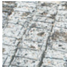
6.1.8 In restoration of the reinforcement cover, high pressure scarification assures adequate adhesion of the interface
