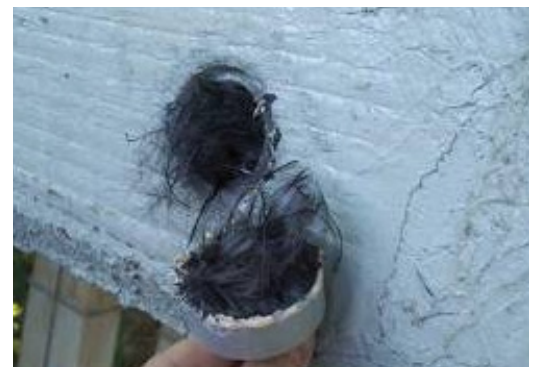
2.5 The pull-out test, manual impregnation is not correct if the fabric is heavy weight
